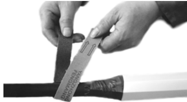
Abrade the cable sheath circumferentially on the cleaned area with the abrasive strip
