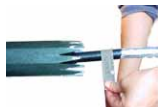
Abrade the cable sheath circumference on the cleaned area with abrasive strip.
